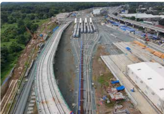
MRT-7 - Depot Facilities, Manila, Filipinas
